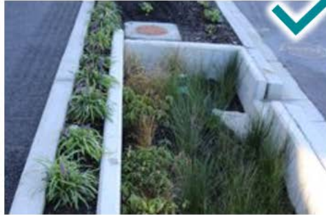
Green drainage elements
