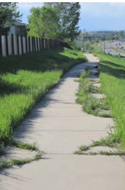
◀ 3.4.1.12: Cracks and weed growth are quickly diminishing the viability of this path segment.
