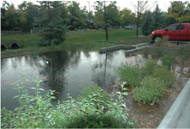
Typical bioretention with ponded runoff during rain event
