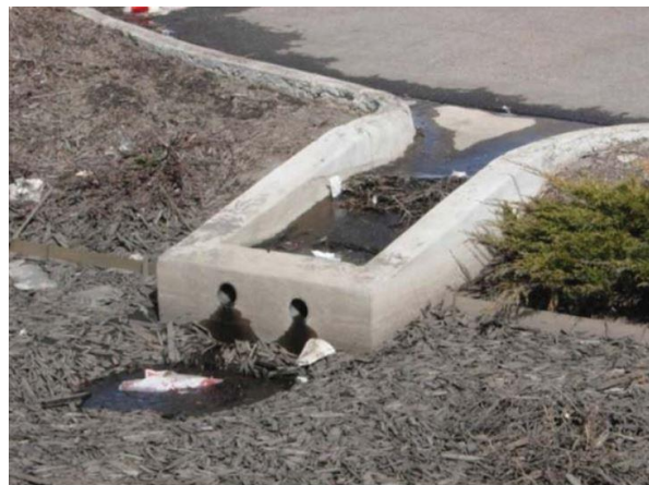
Bioretention forebay that needs sediment and debris removed.
