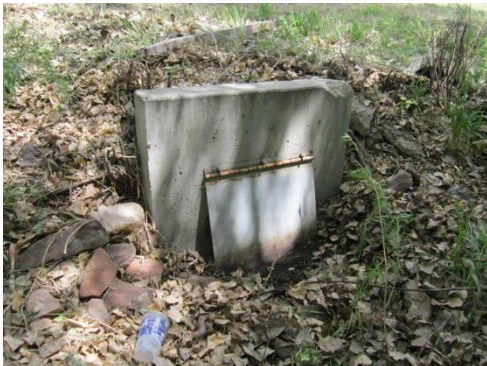
Poorly maintained BMP outlet structure
