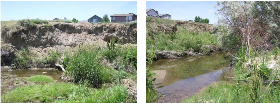
Figure 42. Photos taken in June 2004 showing bank erosion along Big Dry Creek within the Martin and Starika Open Space parcels.
