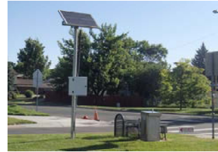
The new solar powered weather station and controller. (weather station not shown)
