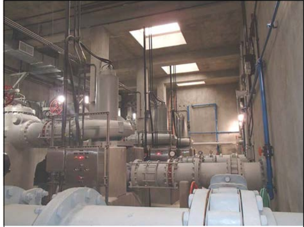
Blower room at the Big Dry Creek Treatment Facility
