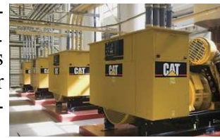
Typical packaged CHP generators
