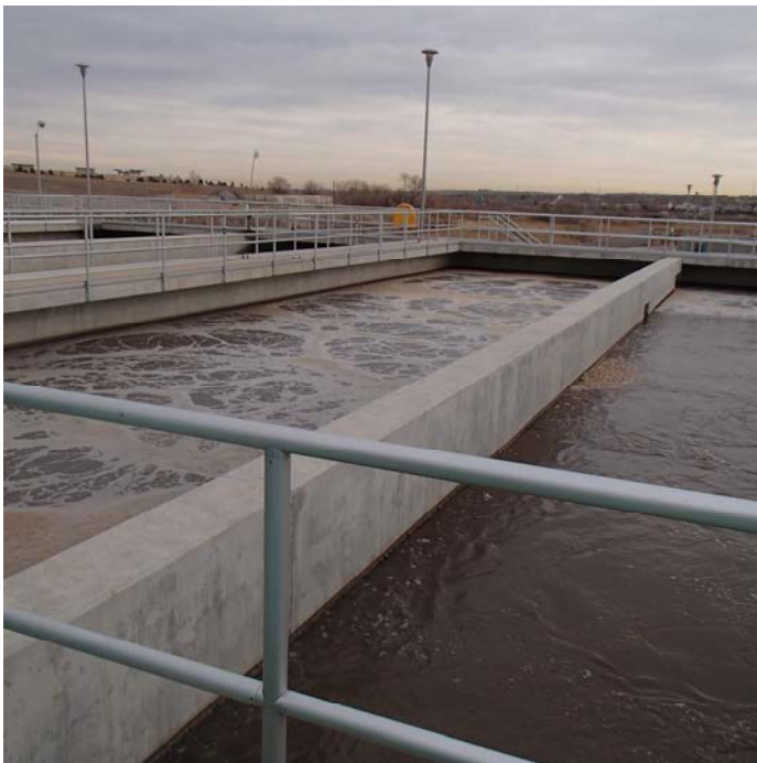
Blower aeration at Big Dry Creek Waste Water Treatment Facility creates conditions favorable for proper waste treatment
