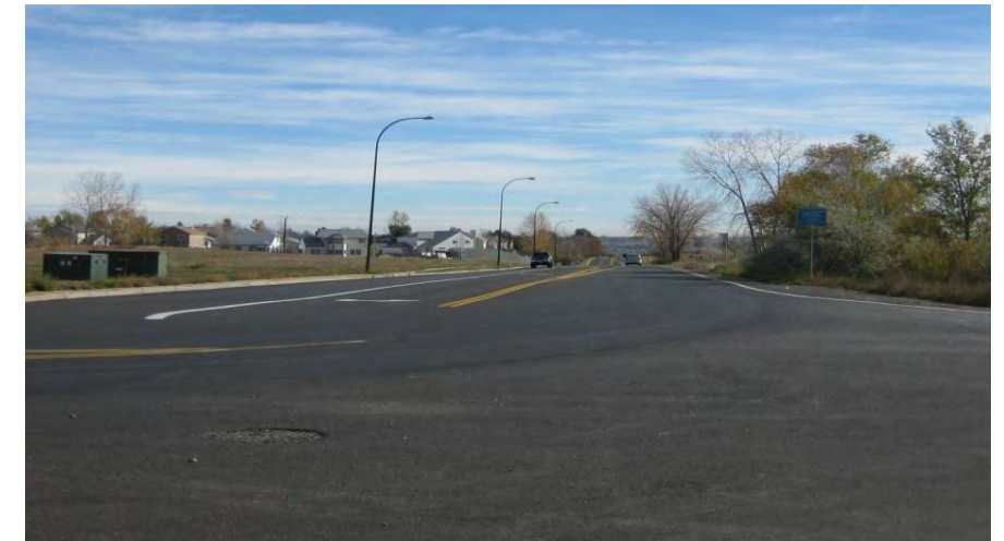
Image 5. The non-standard intersection configuration and lack of pedestrian facilities at West 100th Avenue and Simms Street creates a safety concern for pedestrians and bicyclists during busy summer months
