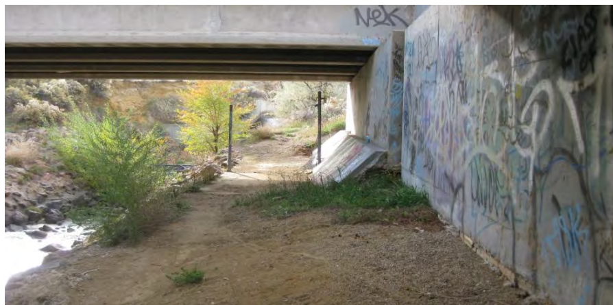
Image 4. Existing social trail under 86th Parkway; a grade-separated crossing requires additional design considerations
