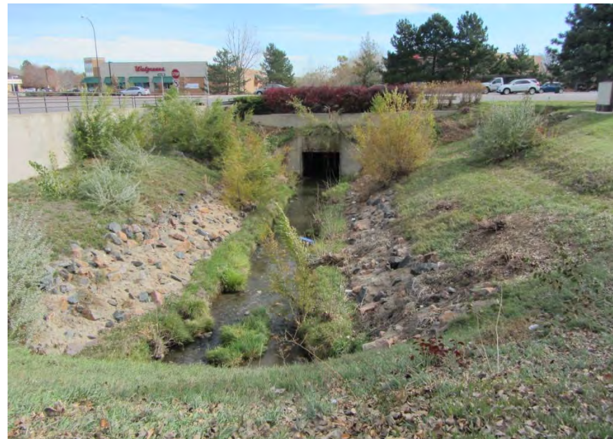
Image 1. The existing box culvert for the Little Dry Creek drainageway under Wadsworth Boulevard
