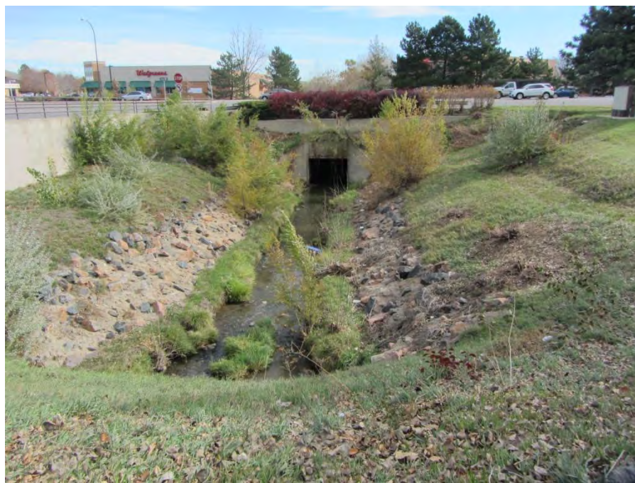
The existing box culvert for the Little Dry Creek drainageway under Wadsworth Boulevard
