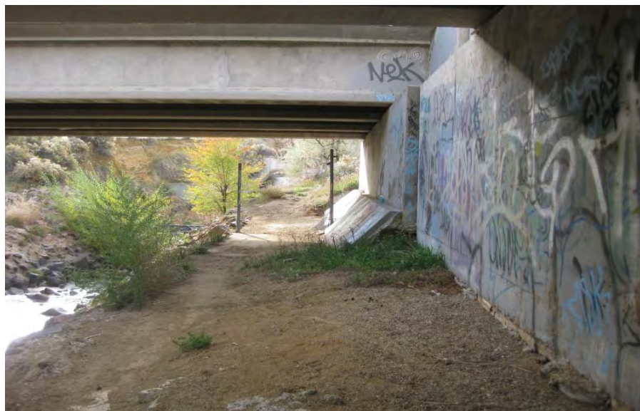
Social trail under 86 th Parkway, which requires additional design considerations
