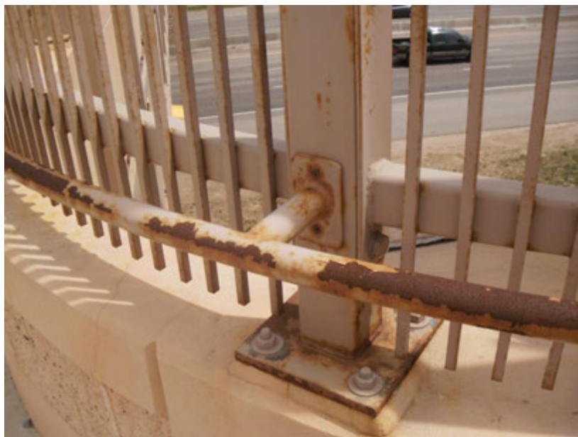
Figure 4. 144th Street coating/corrosion issues
