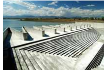
Standley Lake is the primary storage facility for the city's water supply, top. Bottom, the Labrynth Spillway, which is part of Standley Lake Dam.
