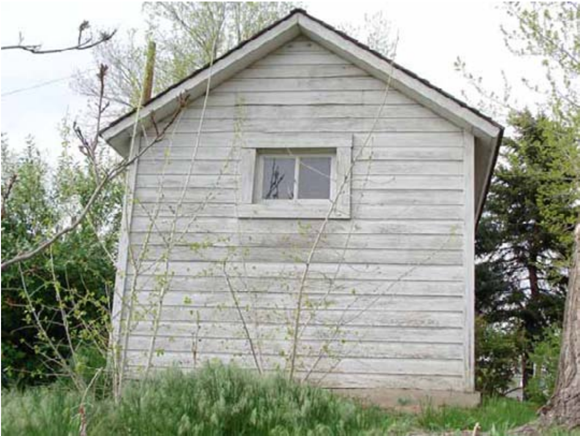
The south elevation has a horizontal window with a simple wood trim. This window does not appear to be part of the original structure.
