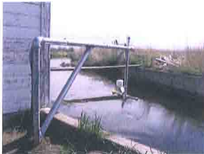
Figure 3: Mounting Arm with Ultrasonic Sensor Attached. Potential configuration should it not be possible to mount ultrasonic underneath existing bridge.
