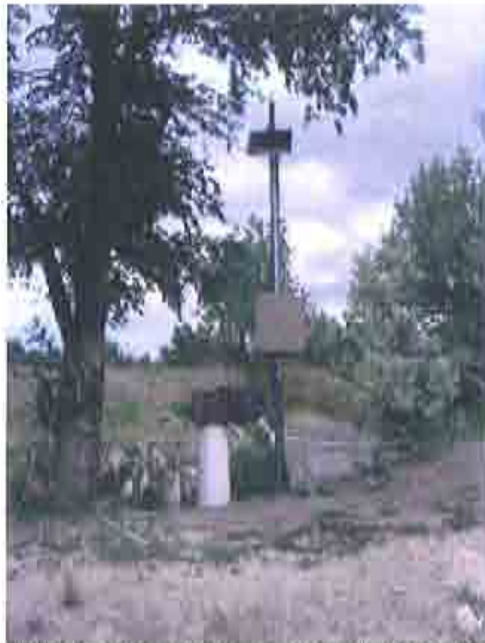
Figure 2: Mast with an Enclosure and Solar Panel Mounted.
