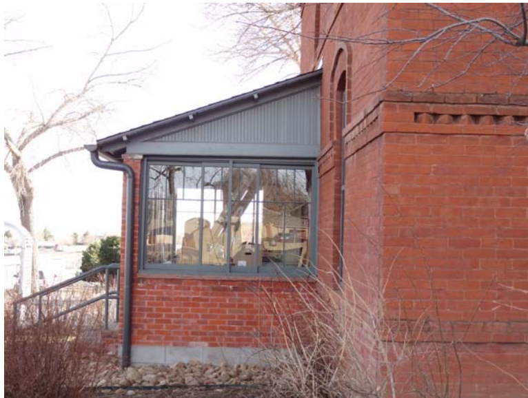
Photo shows east side porch with shed roof, beadboard gable end, sliding wood frame upper windows, brick wall at lower portion of porch, and exposed foundation with parge coat of concrete designed to resemble cut stone.
