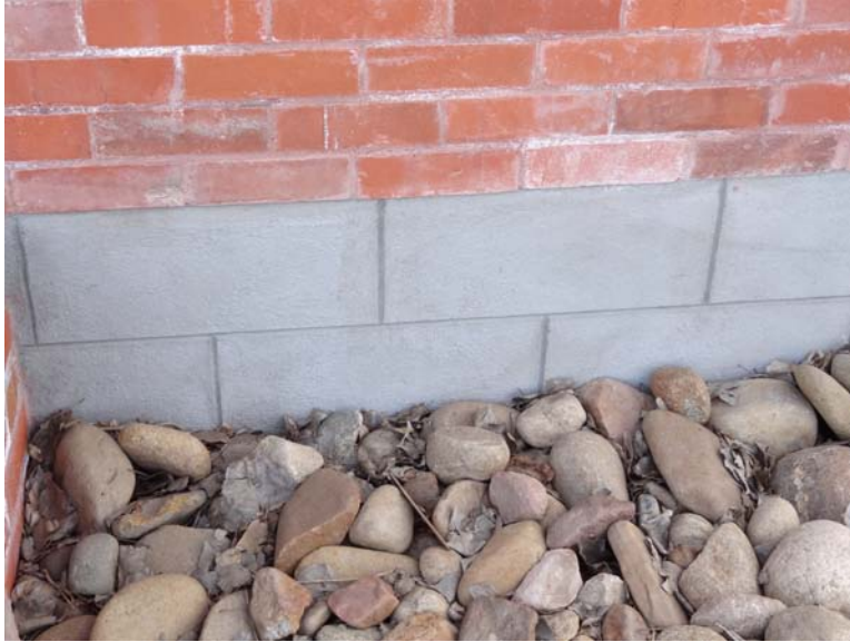
Photo shows detail of restored concrete parge coat on foundation with design to resemble cut stone.
