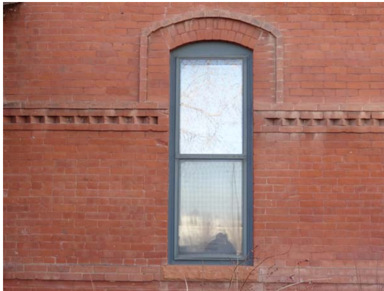
Photo shows typical wood window with 1 over 1 sash, arched decorative brick above window and stone sill. Decorative horizontal brick bands at sill and midway at upper sash are typical.
