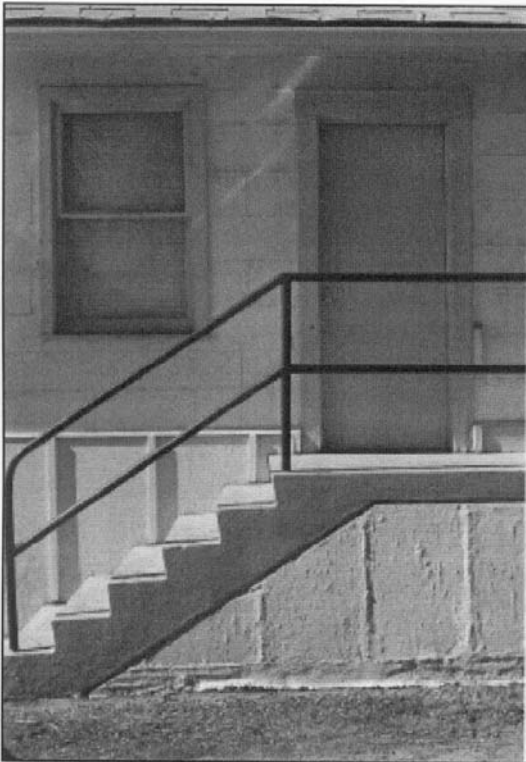
Photo No. 5: Rear Stairs/Typical Window The Rear Door, stairs and railing (serving as an exit from the stage) and a typical window are included in this photo.
