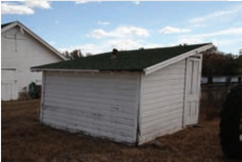
Priority stabilization measures would address structural integrity of the farm buildings, like the brooder house, above
