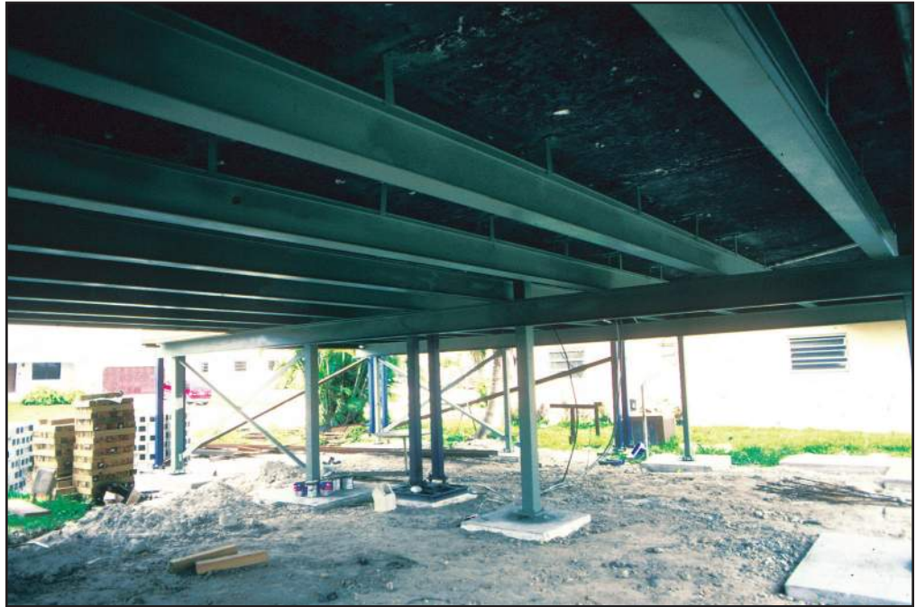
Figure 82 While the jacks and beams supported the house, new steel foundation members were installed below.
