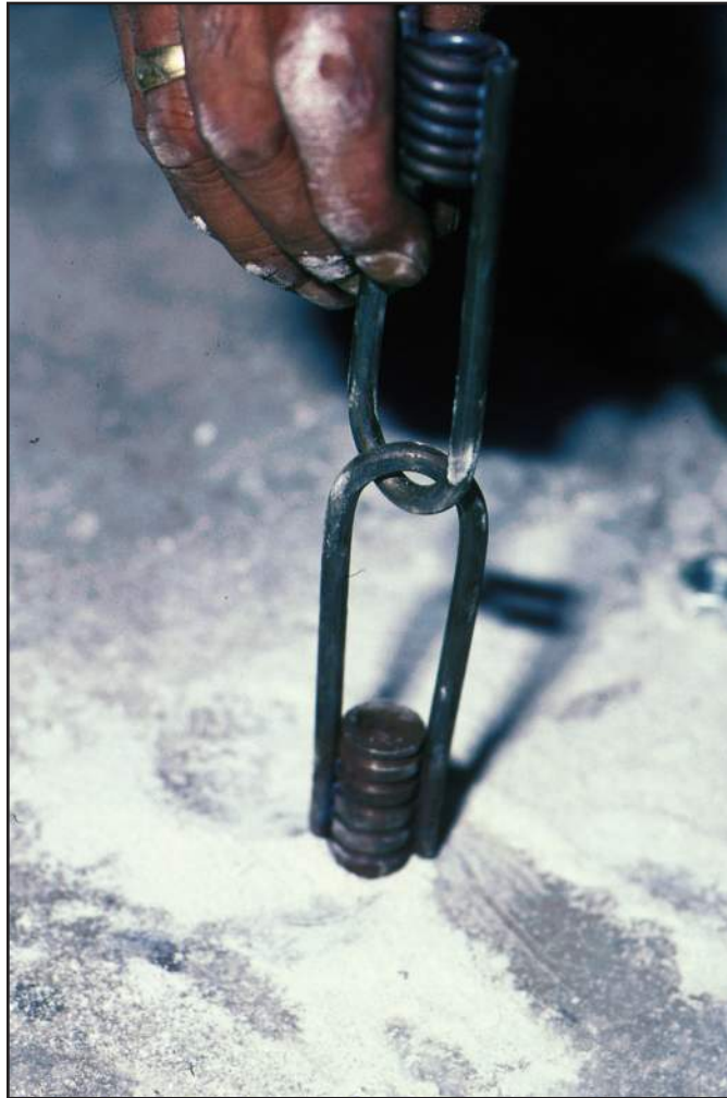
Figure 78 ... and use hangers to attach the anchors to the grid of steel beams.
